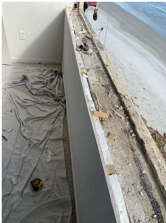
Picture 3: Window sill of Unit 508
