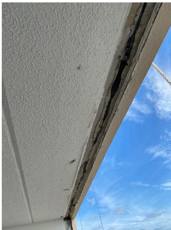
Picture 4: Header of Unit 508
